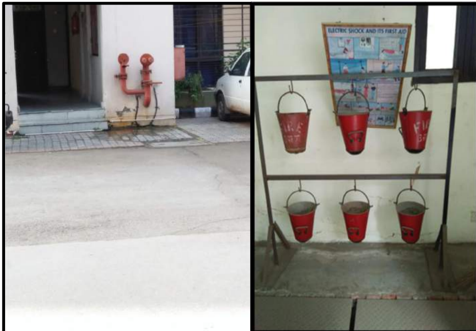
Fire Fighting Equipment
